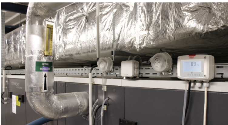
CP210-R in the air handling unit of an industrial facility.
